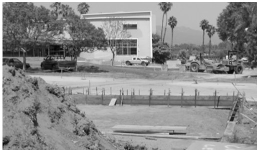
▲ Construction of handicap-accessible parking spaces and passageways at San Marcos High School.
